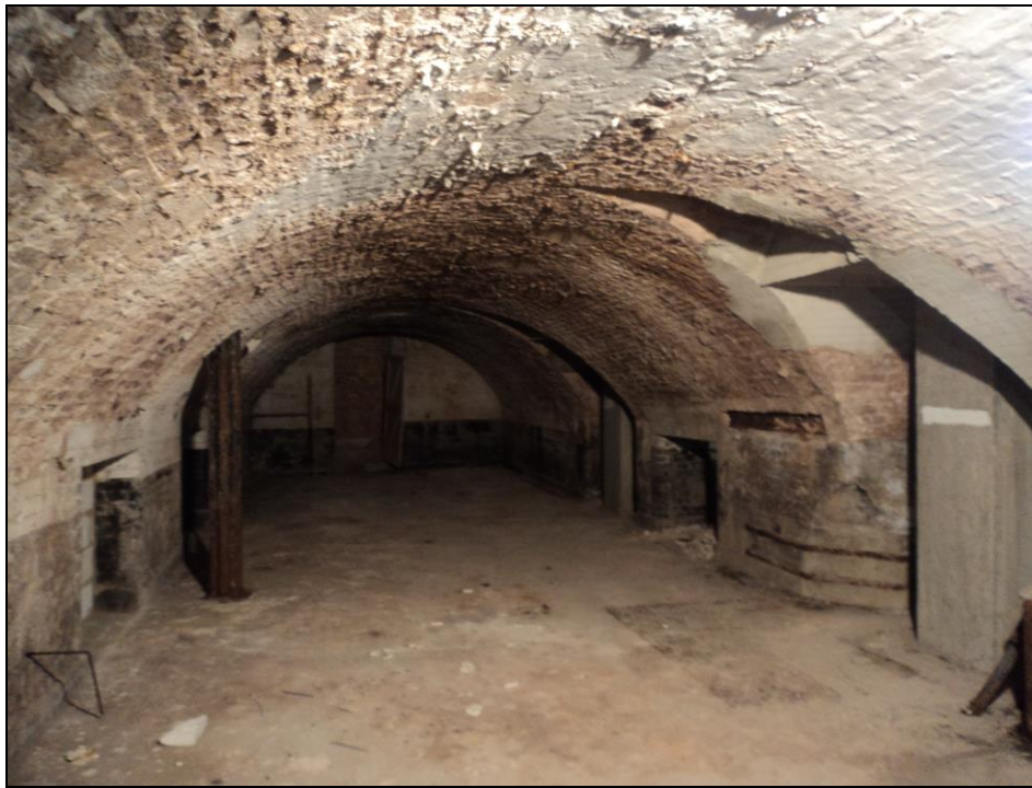
Internal view of existing grade II listed vaults at upper basement level.
